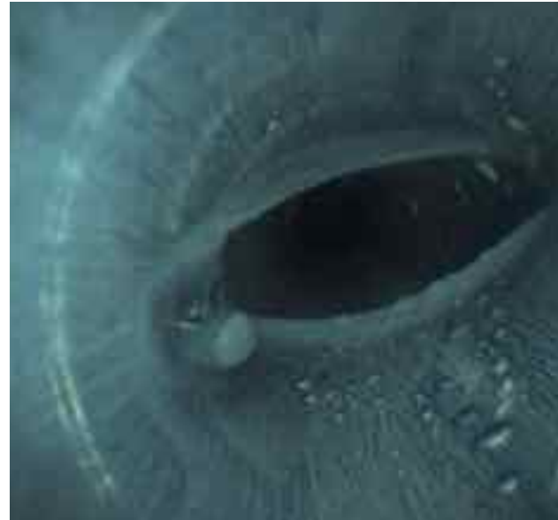
structure damage in the chanel and waterdrops
